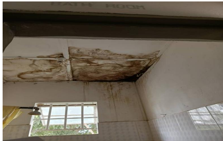
Plate 8: licking roof of the labor room toilet
