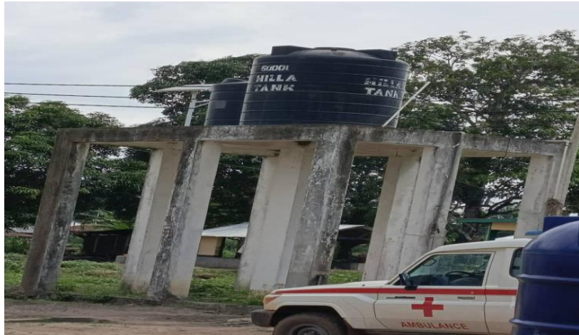
Plate 14: Elevated water storage tank (nonfunctioning)
