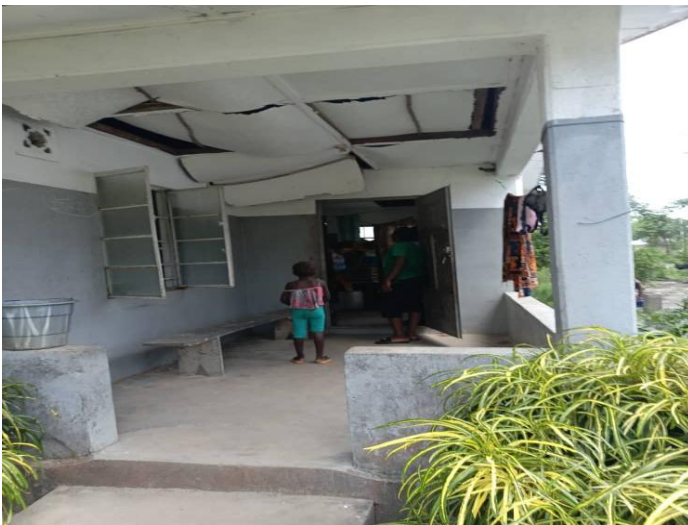
Plate 15: Falling ceiling of staff quarter
